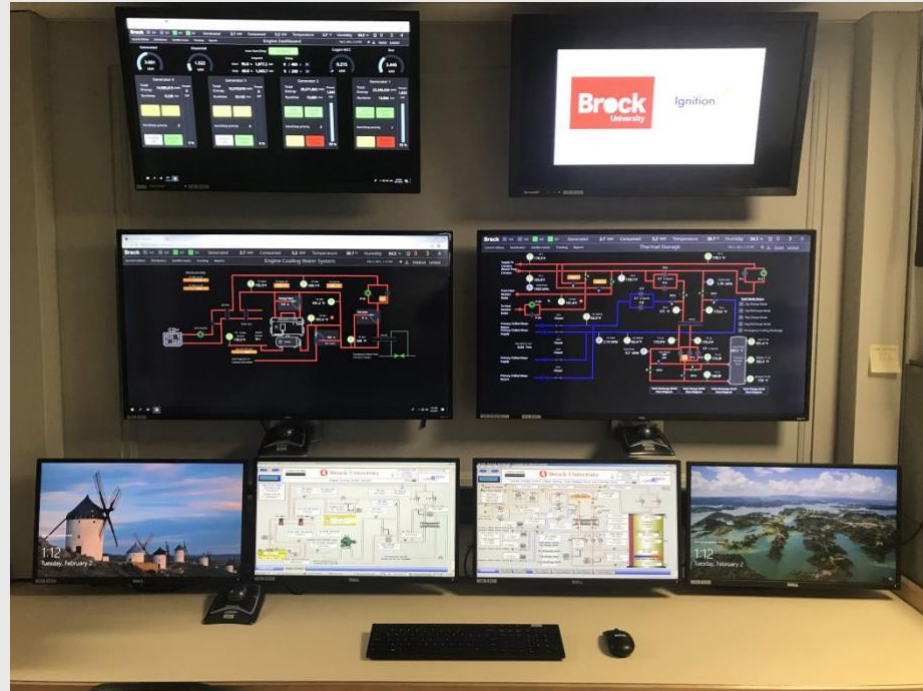
Photograph of the District Energy System's control room.
