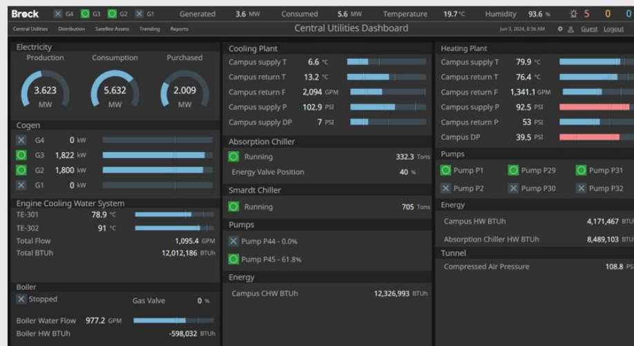
Screenshot of a data-intensive dashboard on SCADA system. Additional data points and screens will be added when adding metering infrastructure.
